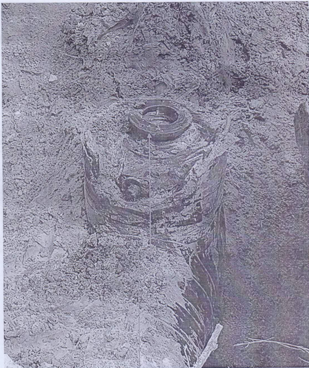
6" VALVE FROM UNKNOWN PERSON ON THE FACILITY
